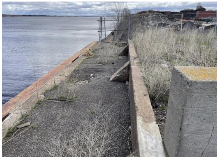
Figure 7: Sinkholes at Duluth Lake Port Dock
